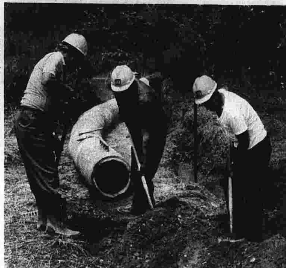
State transportation department workers dig out the path of a culvert being installed on state-owned property at the Burr Corners commuter express bus terminal. Installation of the culvert is a preliminary part of the state's expansion of the commuter parking lot to 330 parking spaces. (Herald photo by Bevin)
